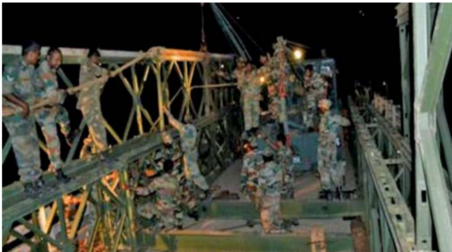
BRIDGING THE GAP Army Engineers and BRO restore connectivity between Rajouri and Budhal by constructing bridge over Ans river at Kot Ranka
